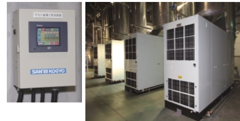
A control panel (left) automatically operates four inverter compressors (right) by varying their outputs between zero and 148 kW.
